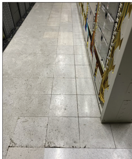
Figure 1: Deteriorating floor in cable company server room
