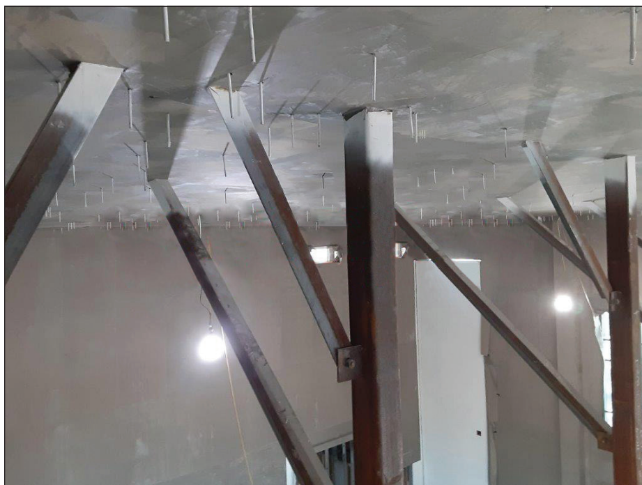
Figure 5: HVAC, electrical, and plumbing support angles with threaded rod penetrating copper fabric shielding material at the ceiling
